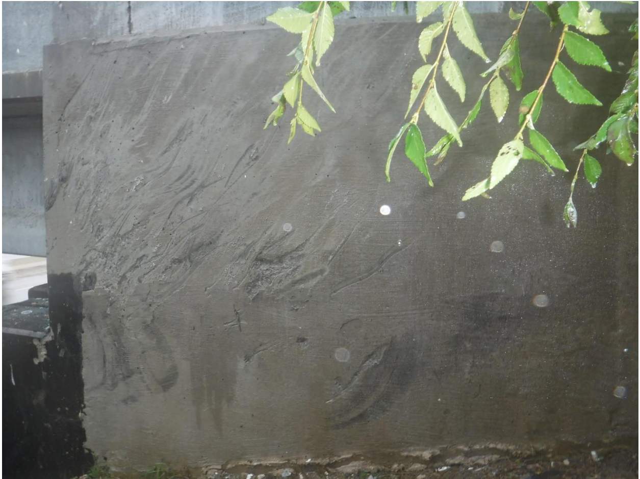
Photo 3: Impacted Wingwall – Surface Abrasions on Concrete
