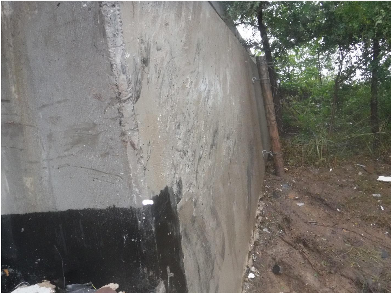
Photo 4: Minor Surface Damage to Concrete
