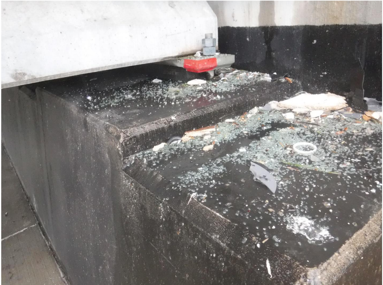
Photo 5: Crash Debris. Bearings Not Impacted
