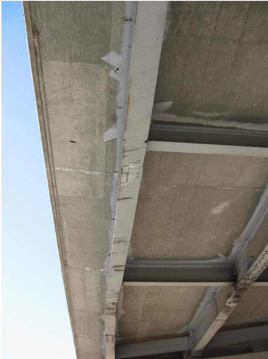
Photo 4: Beam 1 – Damaged Bottom Flange and Web (Out of Plane Bending)
