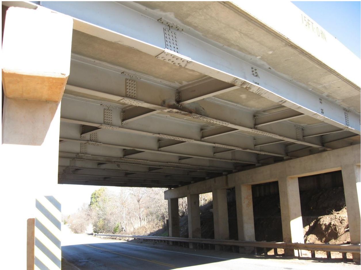
Photo 5: Beam 1 – Damaged Bottom Flange (Out of Plane Bending)
