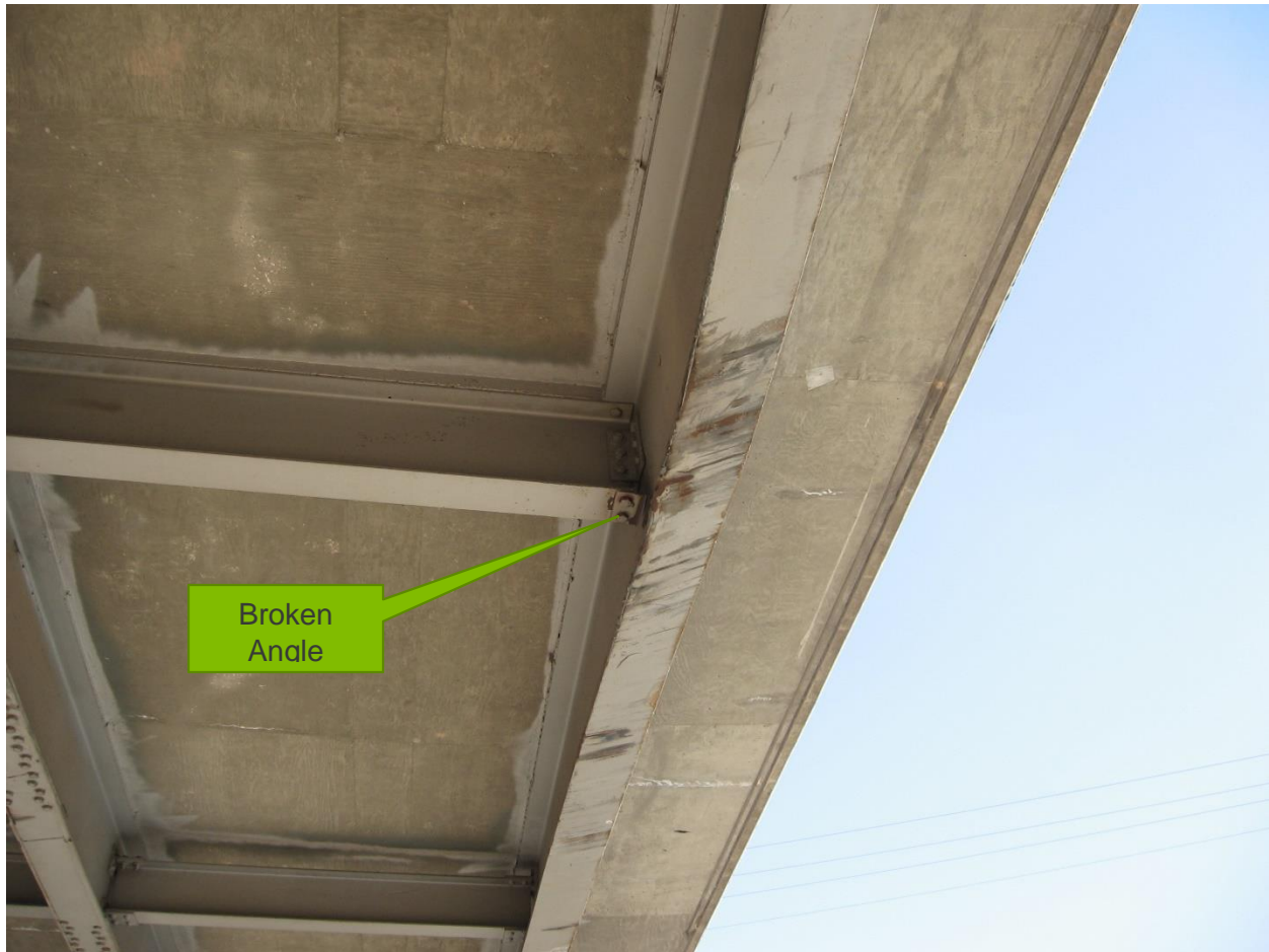
Photo 3: Beam 1 – Damaged Bottom Flange and Diaphragm Connection
