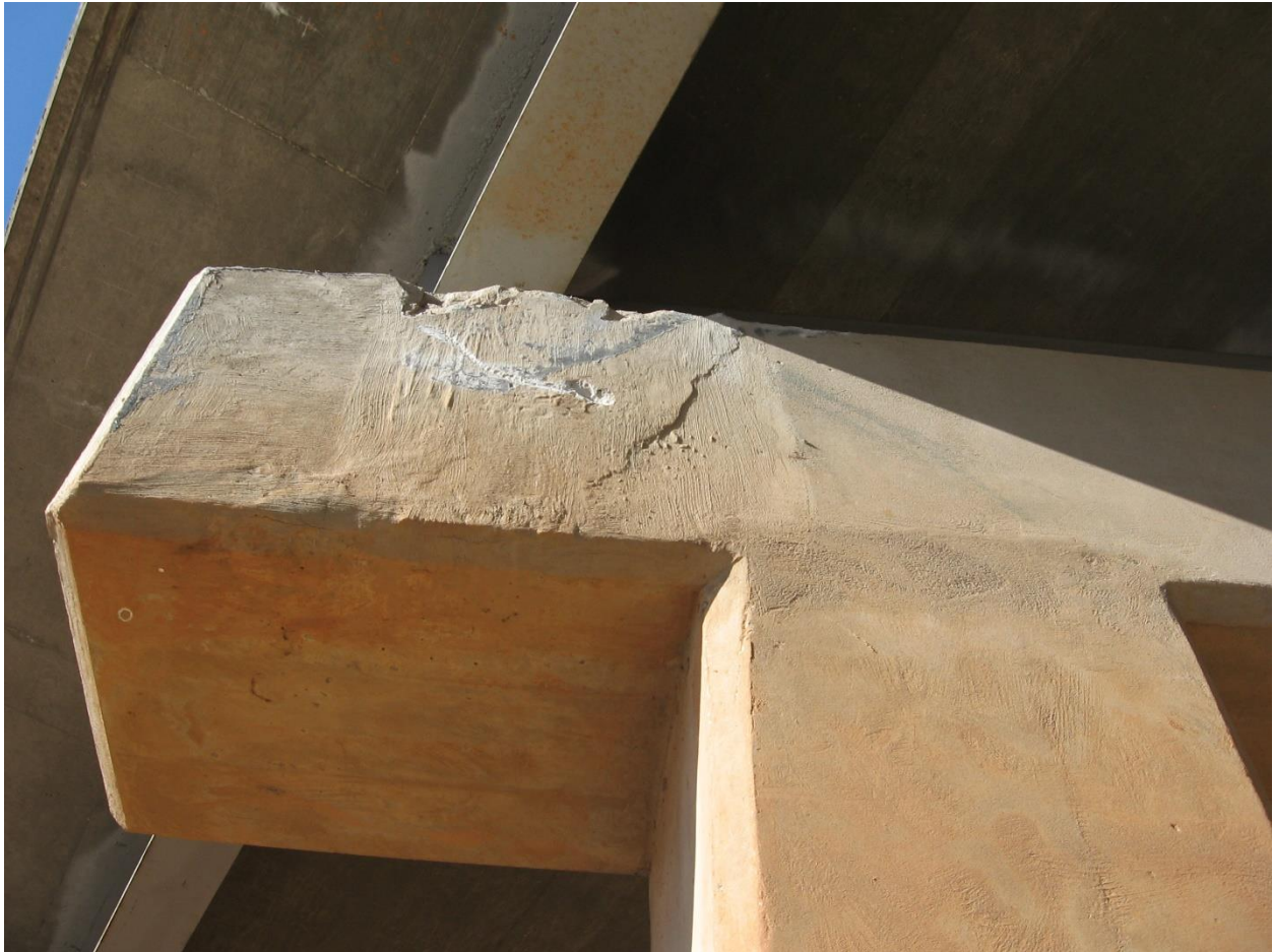
Photo 9: Pier 1 – Damage to the Cantilever at Beam 1 Bearing
