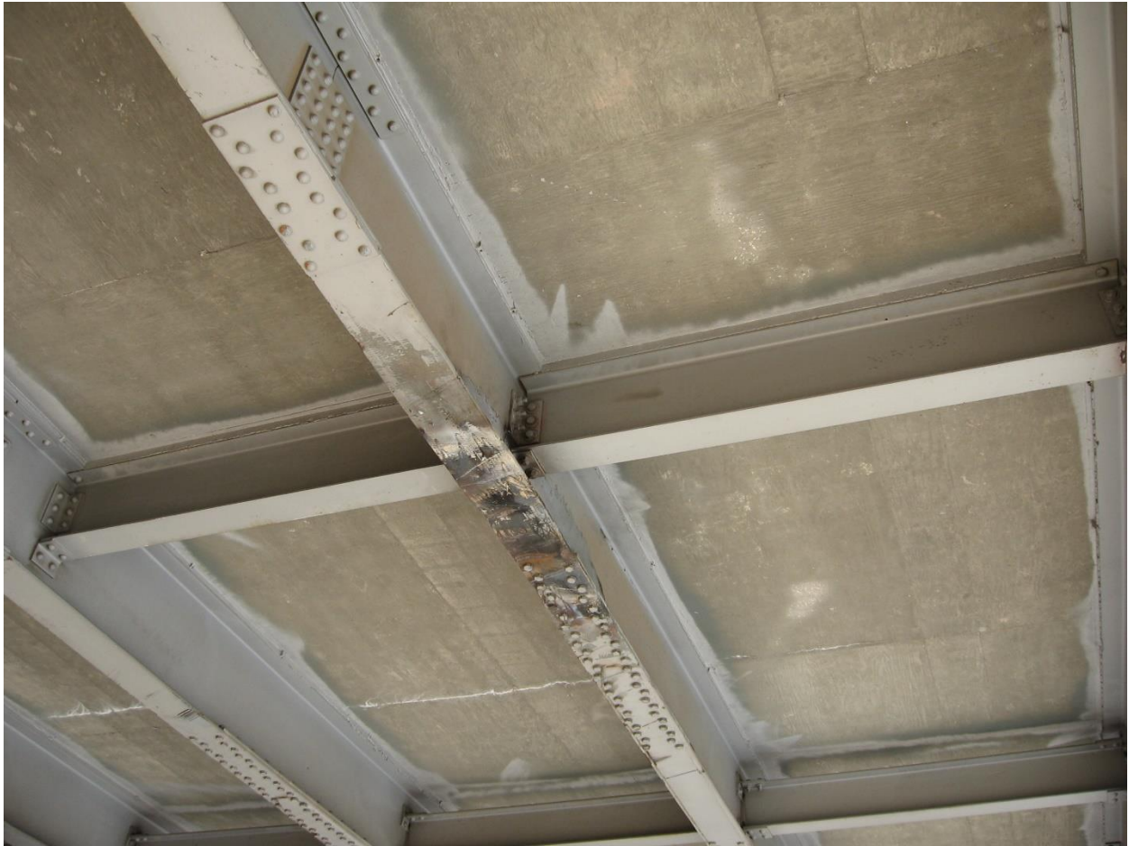
Photo 7: Beam 2 – Damage to Bottom Flange, Cover Plate and Diaphragm
