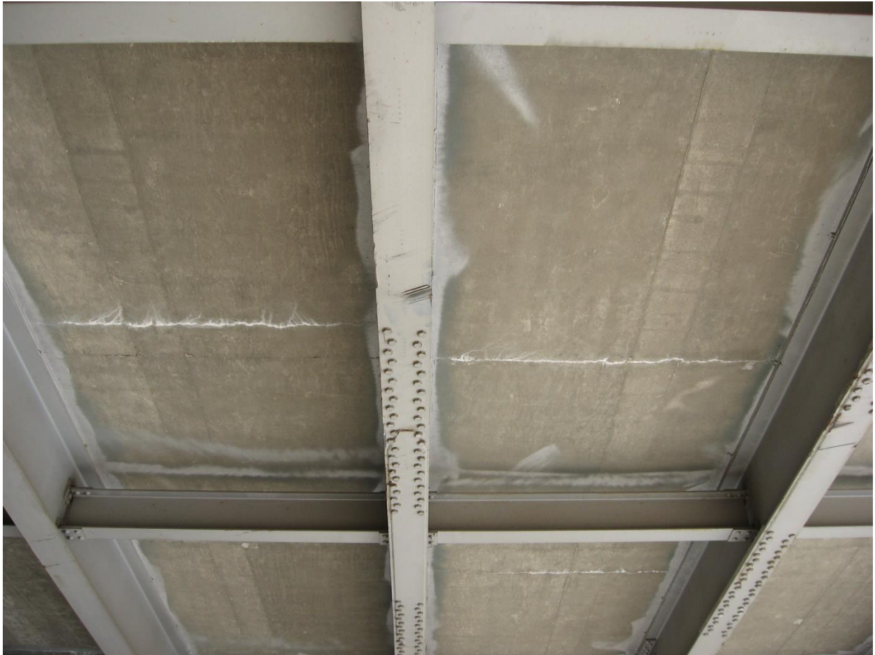
Photo 10: Beam 3 – Damage to Bottom Flange
