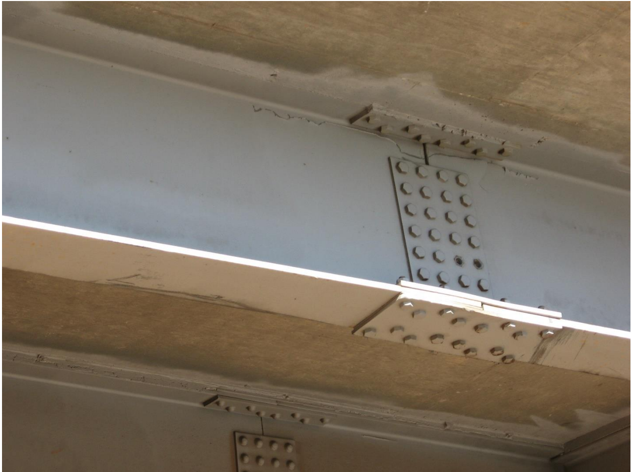
Photo 6: Beam 1 – Damaged Splice Plate with Missing Bolts
