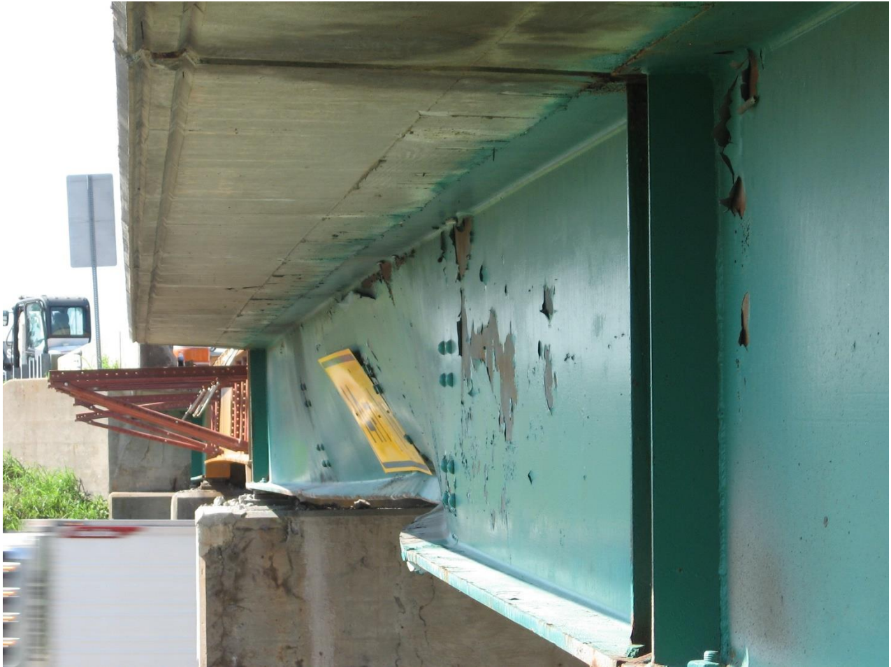
Photo 3: Bottom Flange at point of impact, gouges and deformation.
