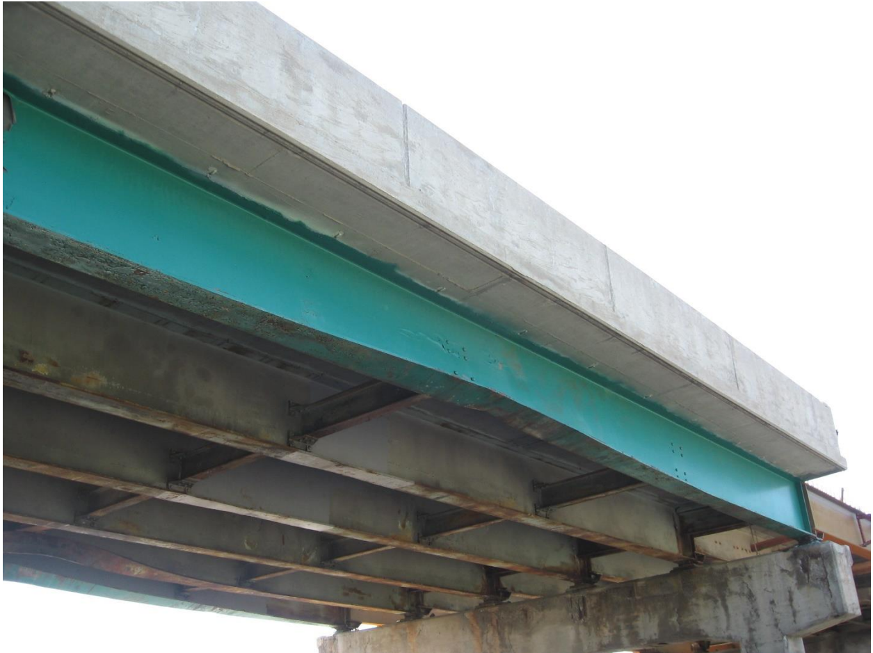
Photo 3: Damage to Beam 6
