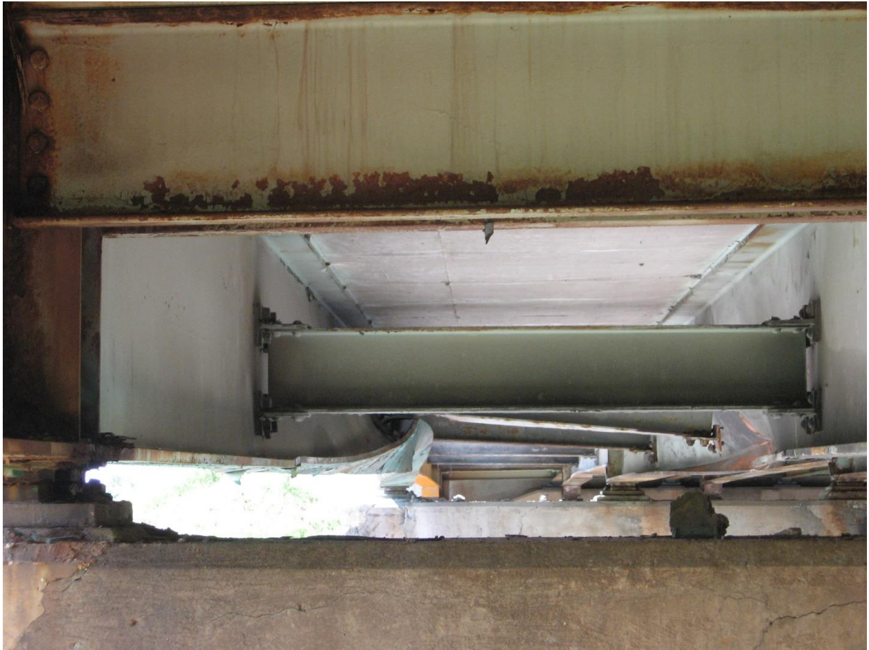
Photo 4: Bottom Flange Deformation. Lateral Displacement. Detached Diaphragms.
