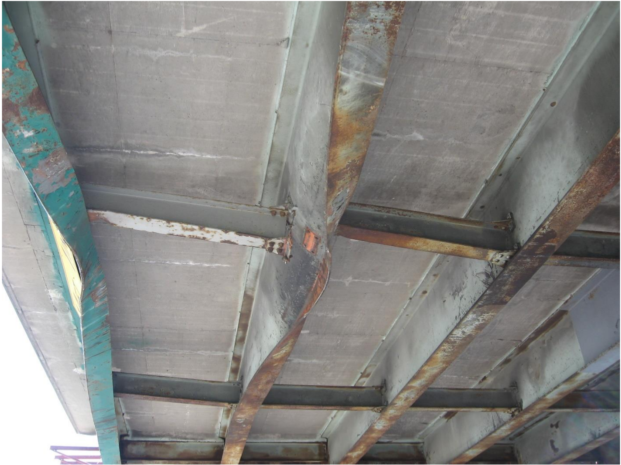
Photo 2: Underside of Bridge. Damage to Beam 1 and 2. Damage to Diaphragm.
