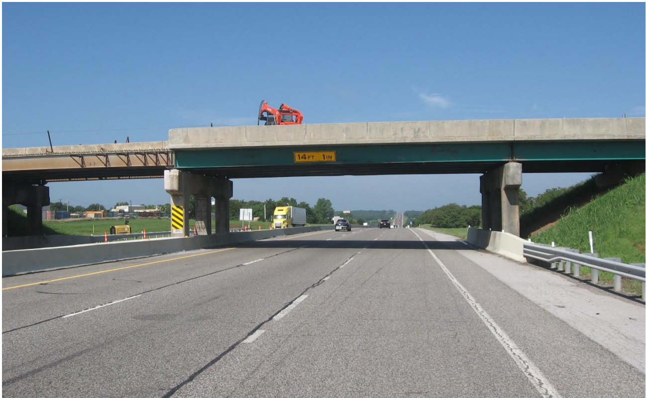
Photo 1: East Exterior Beam. Facing West. Previous Repairs visible.
