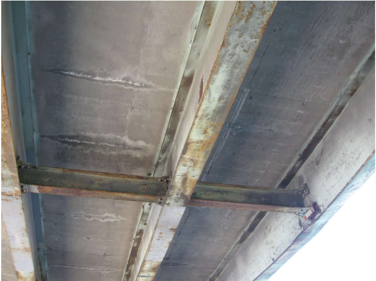
Photo 5: Beam 6 Lateral Displacement and Diaphragm Damage.
